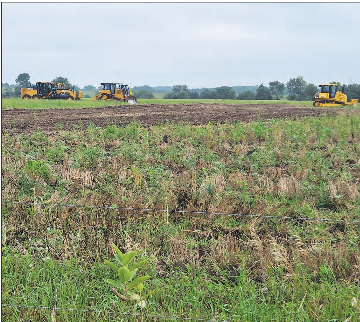
With equipment donated by area businesses and labor donated by Kansas Land Improvement Contractors Association (KLICA), a tile outlet terrace system was installed on SAVE Farm near Riley.
