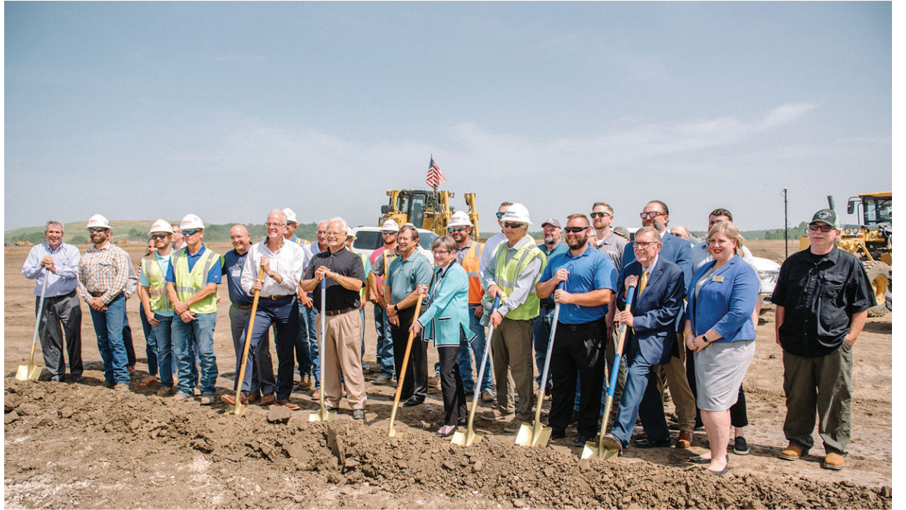
Gov. Laura Kelly was joined by Sen. Jerry Moran and representatives for Roger Marshall as well as Rep. Jake LaTurner along with other state and local officials for the groundbreaking of Bartlett's new soybean crushing plant in southeast Kansas.
