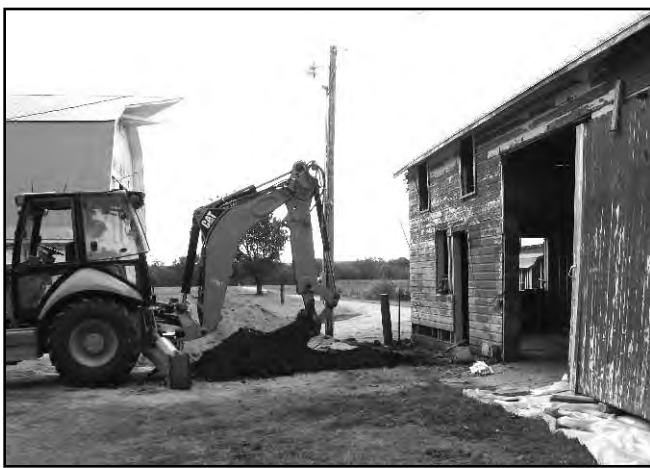
Restoration of a 1916 granary and carriage house has begun to create the Rogler Prairie Heritage Center at Pioneer Bluffs.
