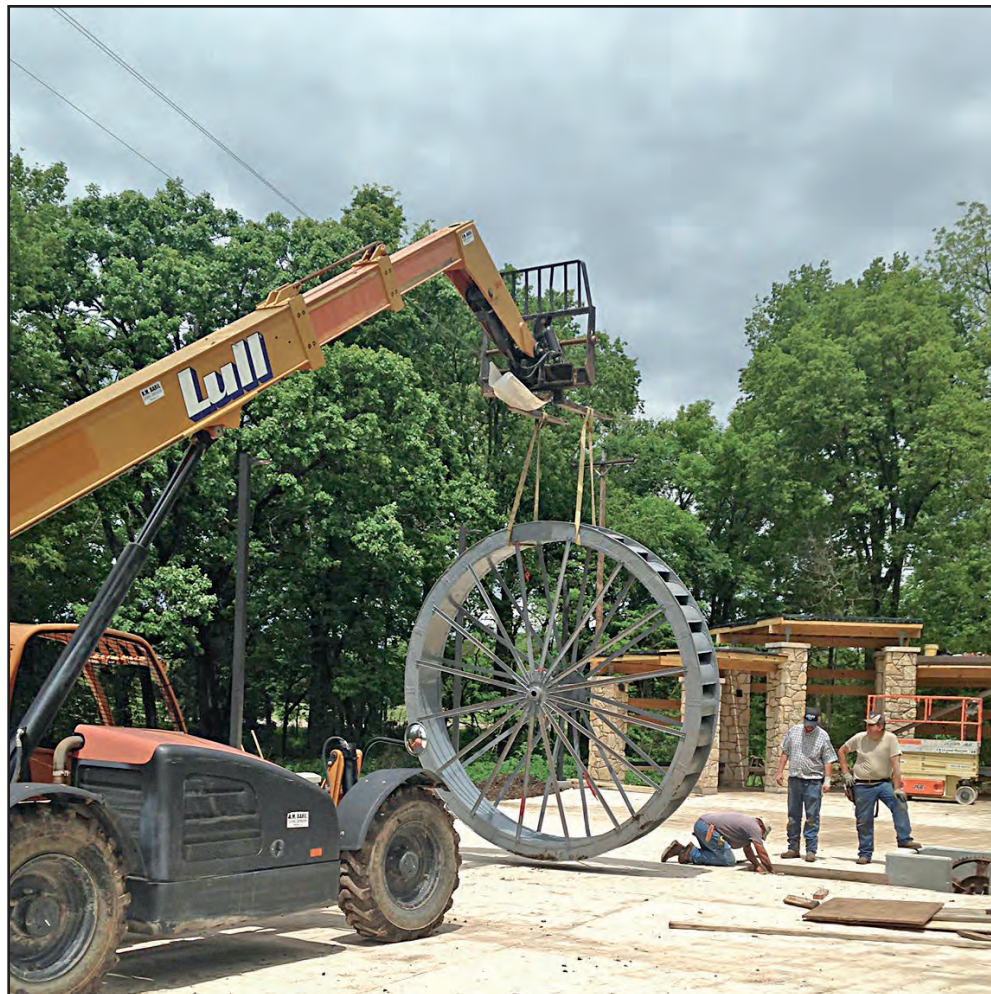
The iconic water wheel was thoroughly refurbished before being set in place.
