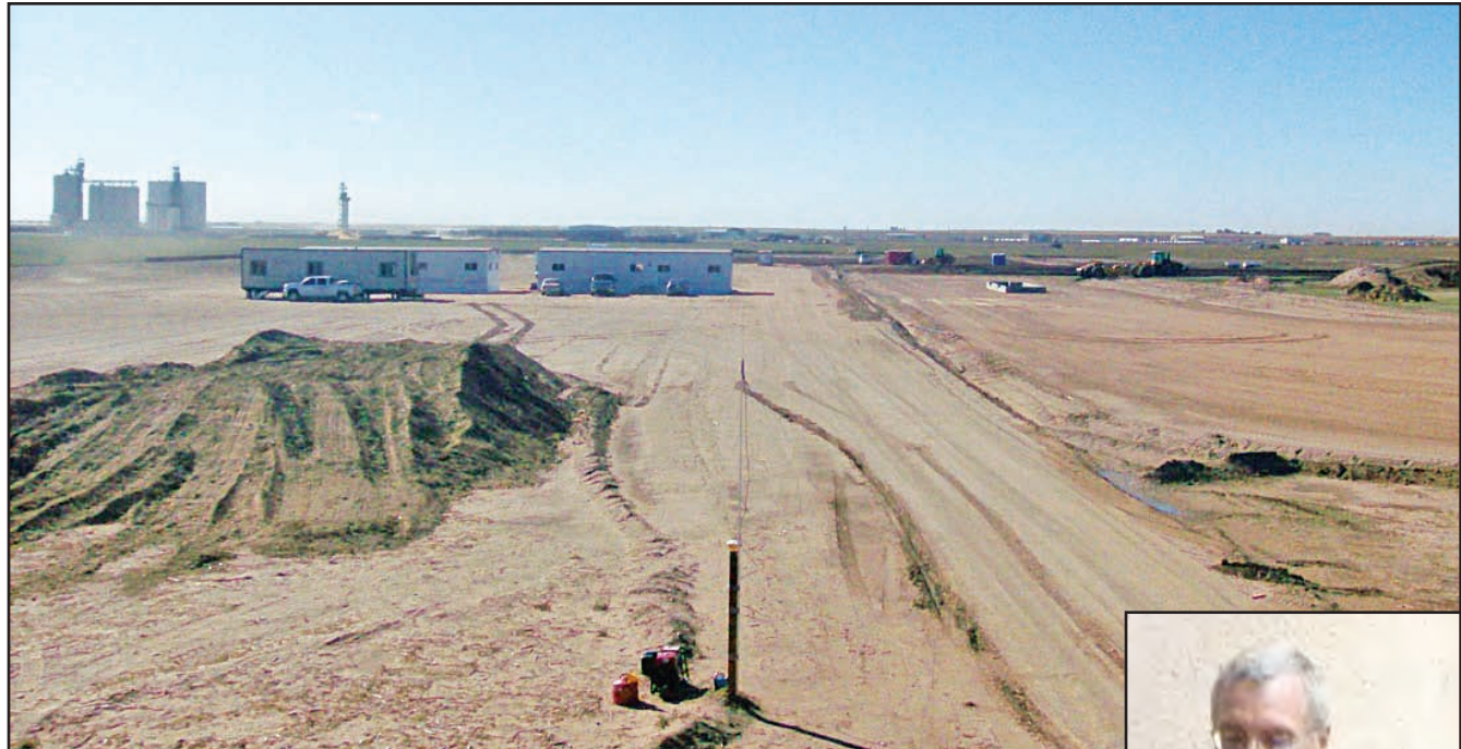
Dirt work has begun for construction of a cellulosic ethanol plant near Hugoton, which is expected to be in full production in late 2013 or early 2014.
